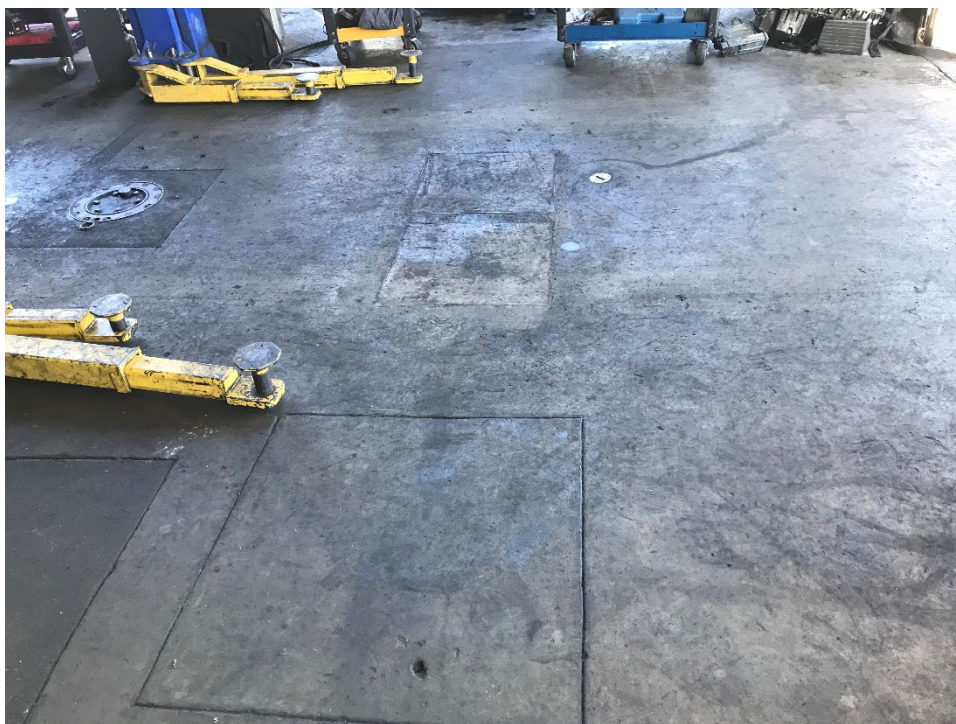
Photograph 14. Patched area inside the auto body shop; possible former clarifier.
