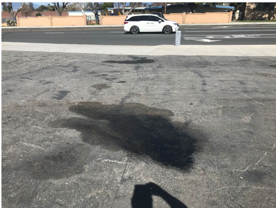
Photograph 20. Staining in the parking area of the Subject Property.
