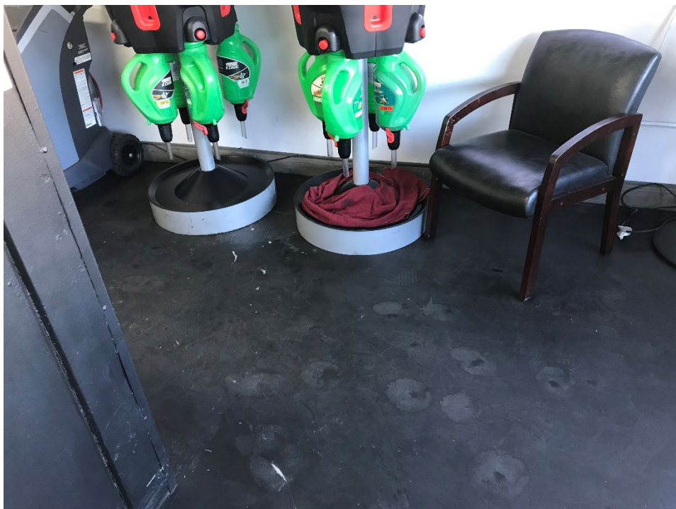
Photograph 10. De minimis staining in the office area of the Subject Property building.
