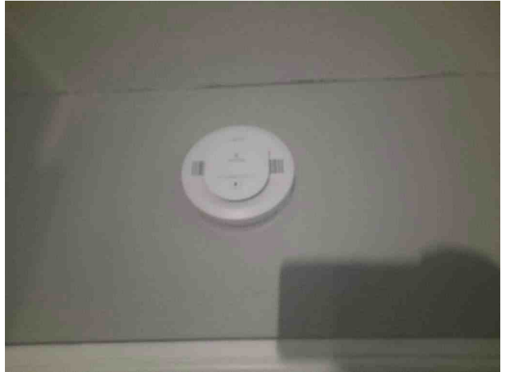
SMOKE DETECTOR - BEDROOM
