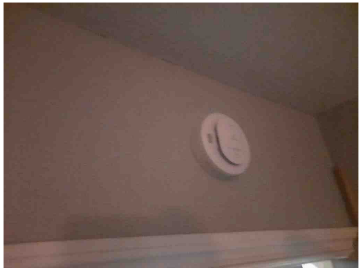
SMOKE DETECTOR - BEDROOM
