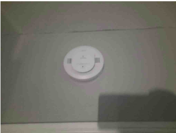
SMOKE DETECTOR - BEDROOM
