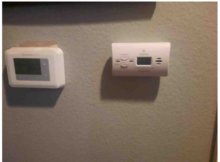
CARBON MONOXIDE DETECTOR HALLWAY ADJACENT TO BEDROOMS
