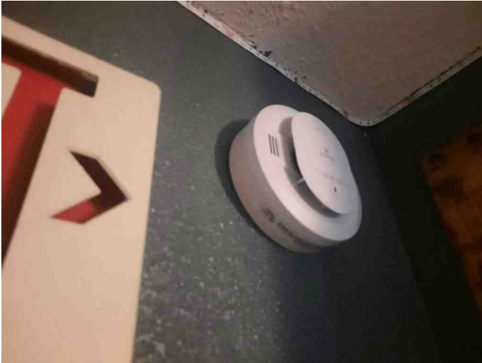
SMOKE DETECTOR HALLWAY ADJACENT TO BEDROOMS
