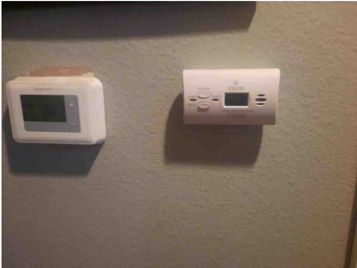
CARBON MONOXIDE DETECTOR HALLWAY ADJACENT TO BEDROOMS
