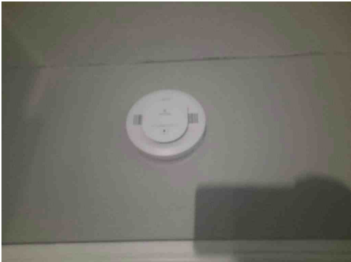
SMOKE DETECTOR - BEDROOM
