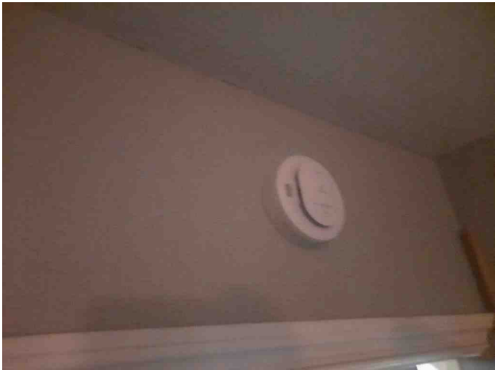
SMOKE DETECTOR - BEDROOM
