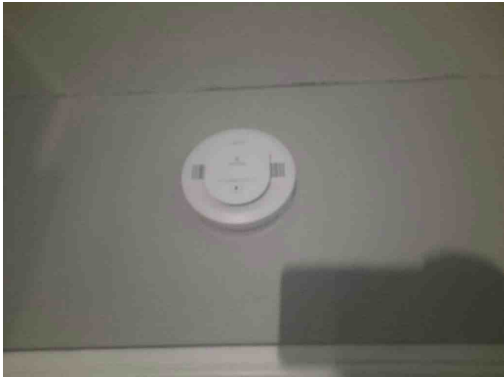
SMOKE DETECTOR - BEDROOM
